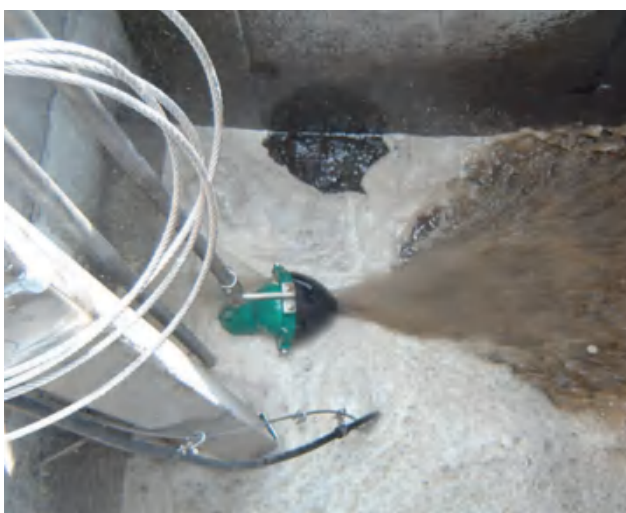
运行中的搅拌喷头 | Agitating nozzle in operation
